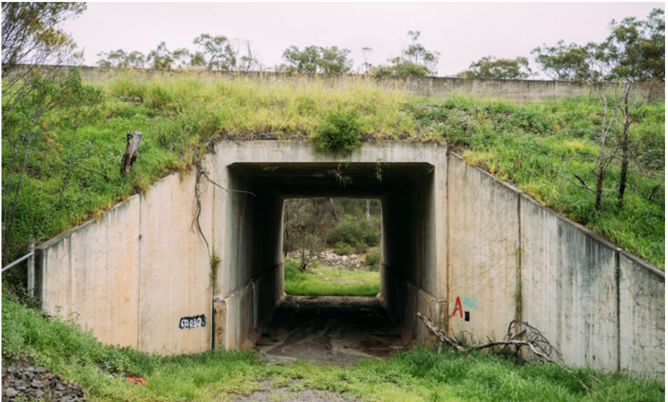
A concrete culvert allows fauna to cross safely under Picton Road at Wilton.
