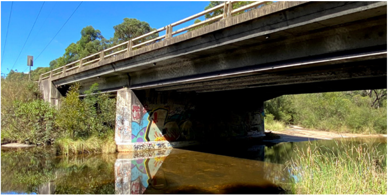
Kings Falls Bridge at Appin Road will be retrofitted to allow safe koala passage under the bridge.
