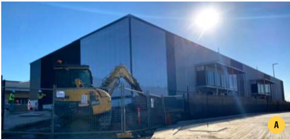
Warehouse units with ancillary office under construction to the northwest of the precinct (Map x.A)
