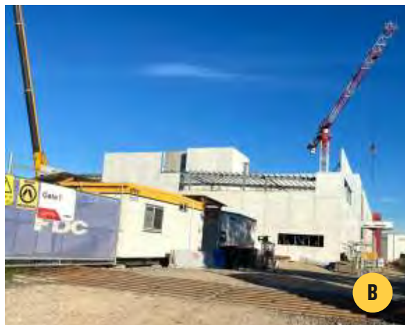
Construction of an additional Digital Realty data centre along Lockwood Road (Map 1.4B).
