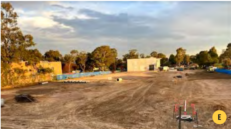
An old newspaper factory site that is being redeveloped. A standalone office warehouse is currently under construction (pictured in the distance) and there plans to build an additional 32 industrial strata units.
