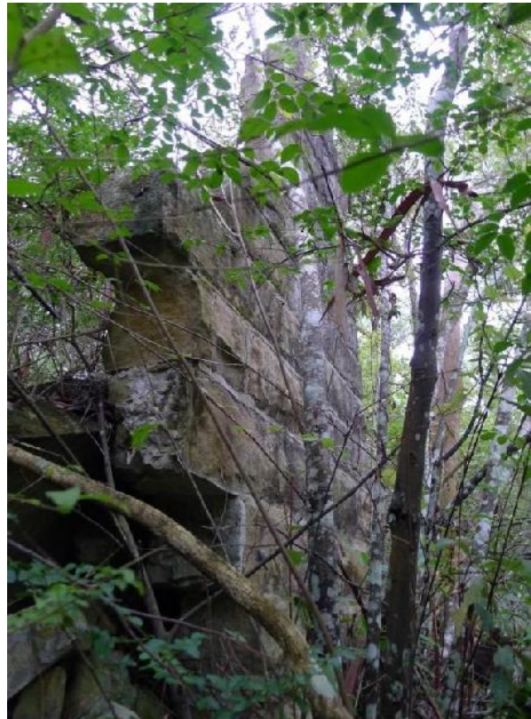
Figure 3.12 Detailed view of a second sandstone wall relating to the Powderworks, believed to be part of the original Office and Magazine building. (Source: GML 2014)
