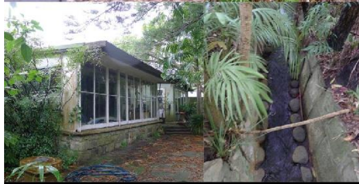
Existing buildings and landscape features from Cicada Glen Nursery (above) could be adaptively reused as elements in the park as landscape features and a cafe. (Source: GML Heritage)
