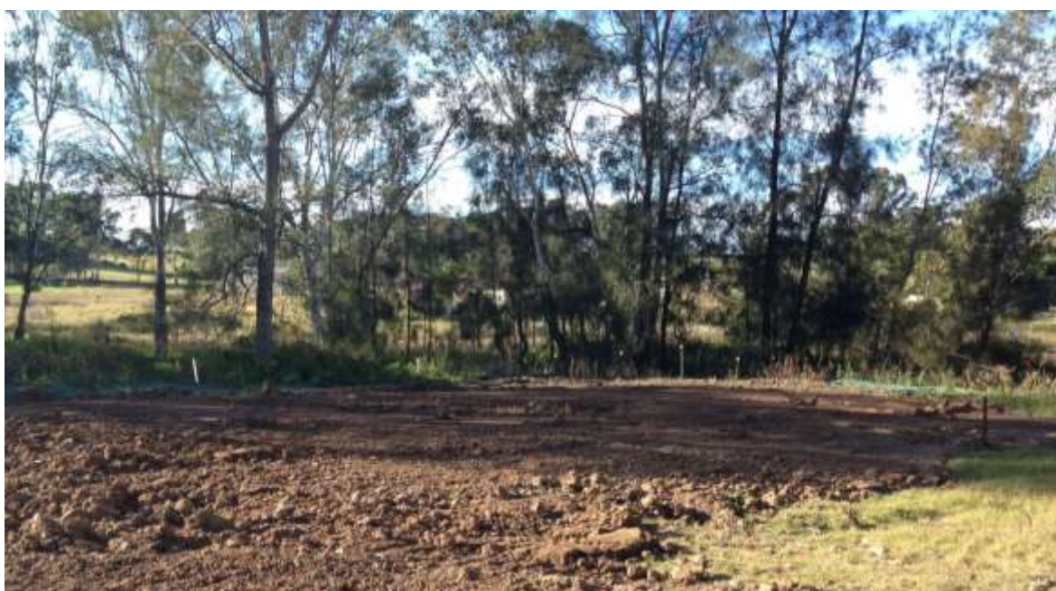
Figure 24. Photograph of disturbance caused by installation of water services in the vicinity of Killarney Chain of Ponds.
