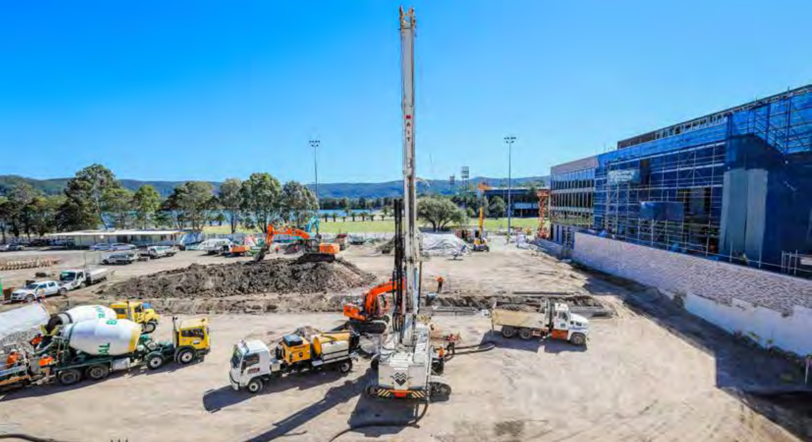
Image: St Hilliers building site in the City South (photo by Salty Dingo)
