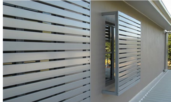
Figure 3-91 Poorly executed privacy screens. These block outlook, sunlight and daylight to windows and reduce amenity of room.
