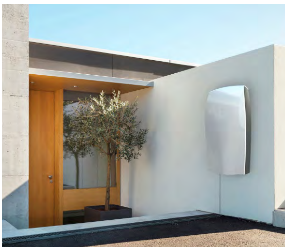
Figure 3-100 Battery storage saves energy generated during the day for use in the evening
