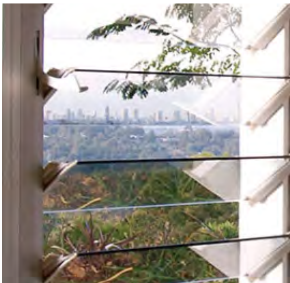
Figure 3-43 Operable louvres allow residents to regulate natural ventilation
