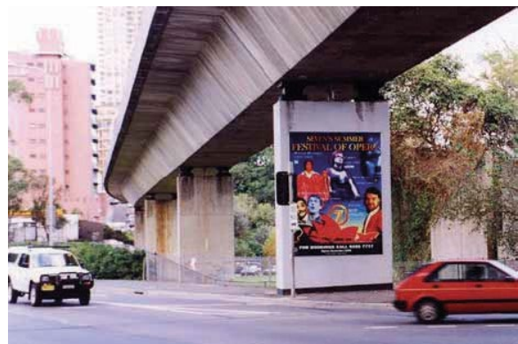
✓ ADVERTISEMENT WITHIN STRUCTURAL BOUNDARIES OF RAIL BRIDGE
