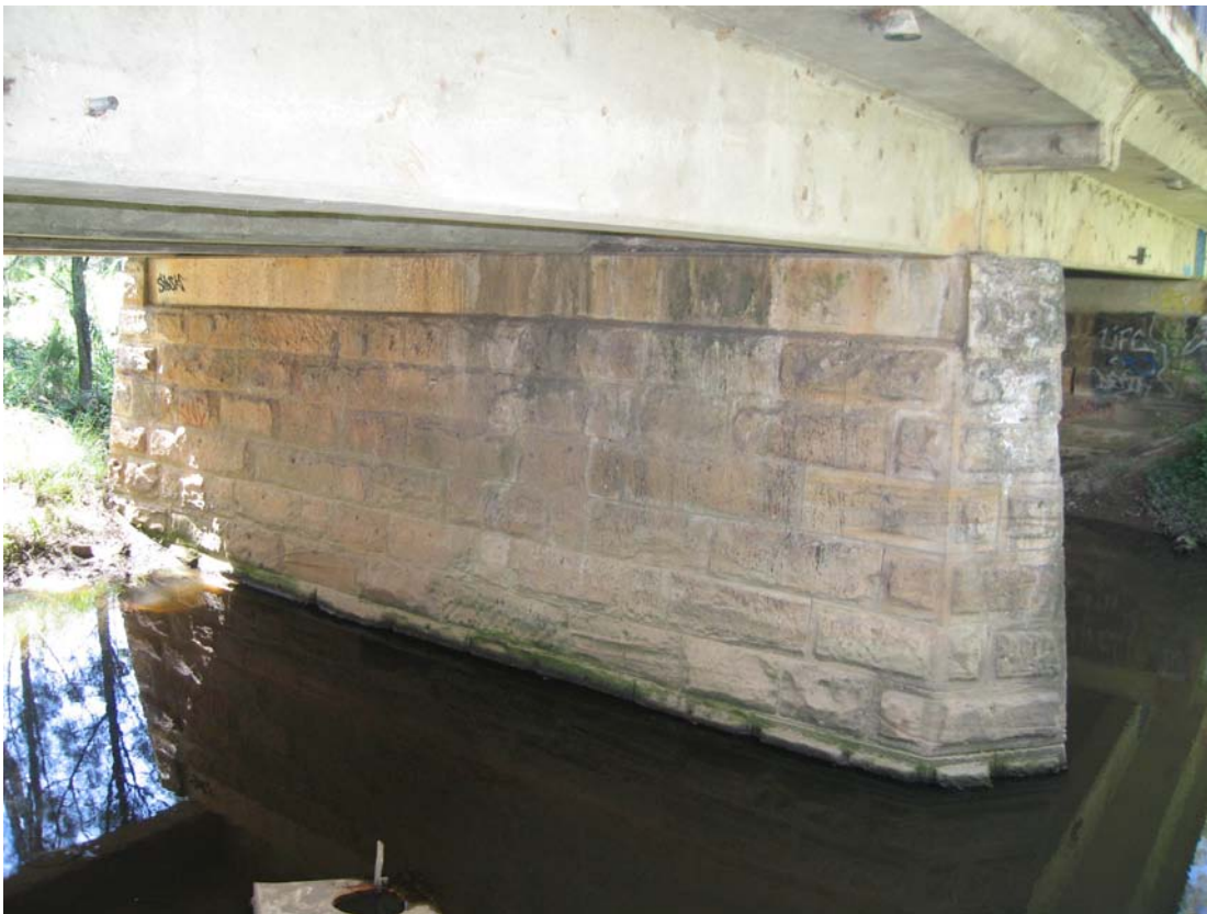
Figure 3.9 View of existing bridge piers across Second Ponds Creek beneath Windsor Road. Note that the bridge is located within the study area. (Source: GML 2009)
