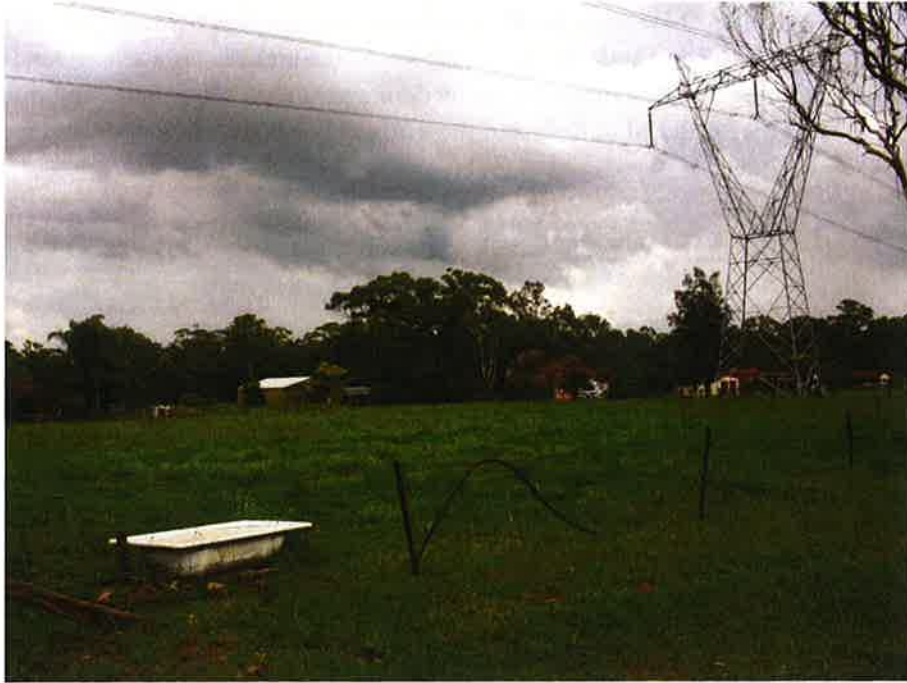
Figure 4.76 Transmission lines leading from the Kemps Creek Substation; view from Boyd Street.
