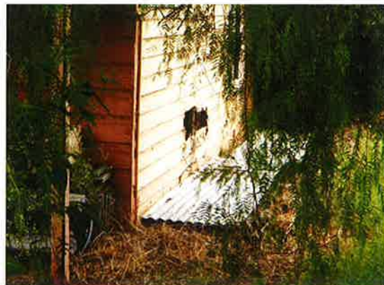
Figure 5.193 Detail of the east elevation showing termite damage.
