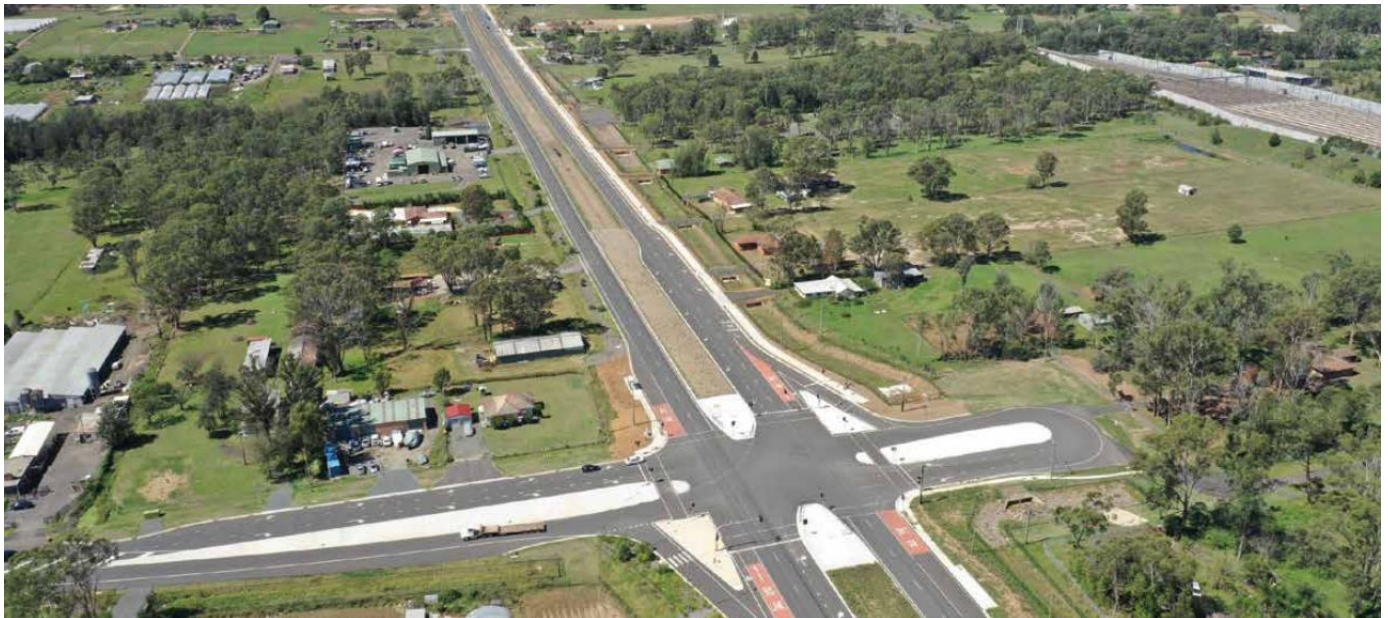
Bringelly Road upgrade from King Street looking east towards Leppington. RMS community update November 2019 .
