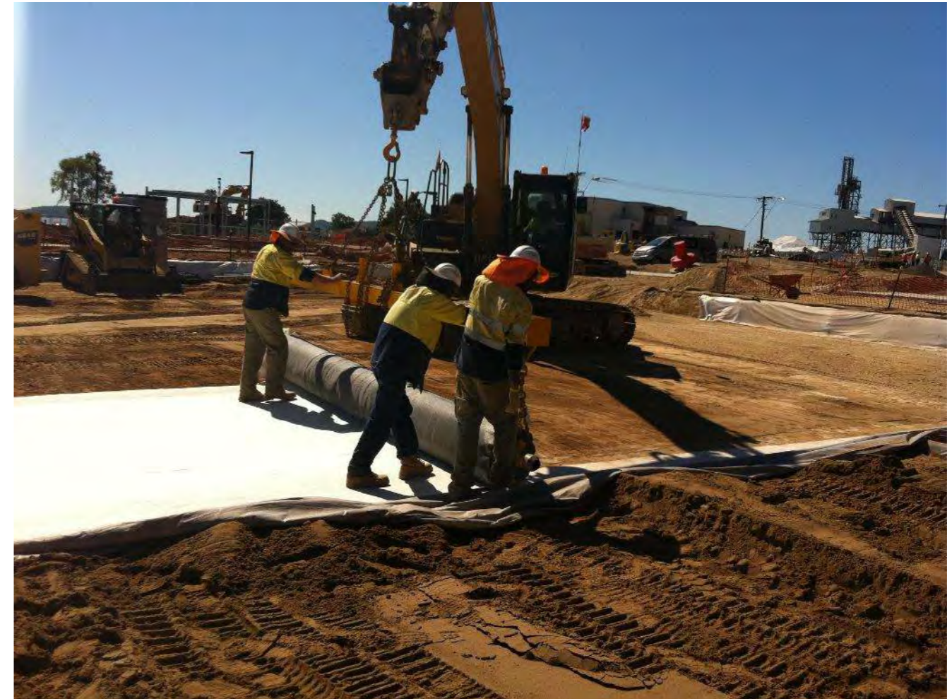
Installation of a waterproof liner to create below ground storage for a grassed open space area in Queensland (E2Designlab)
