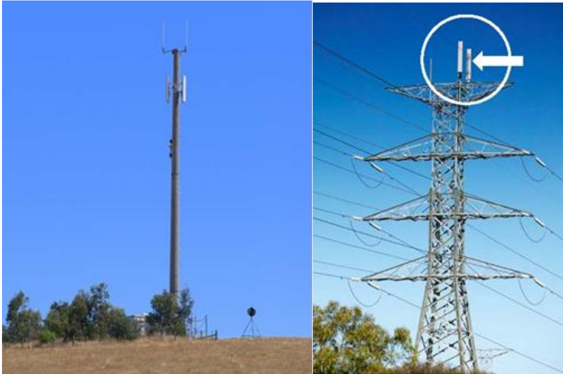
Figure 5 Macrocell base station antennas co-located on an existing high voltage tower
