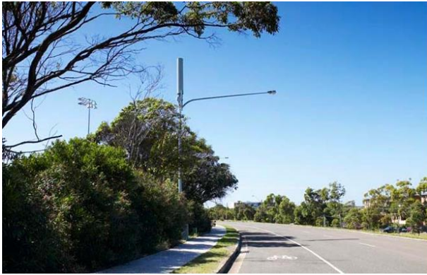
Figure 3 Panel antenna on street light pole
