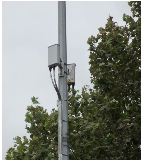
Figure 6 Microcells attached to a light pole.
