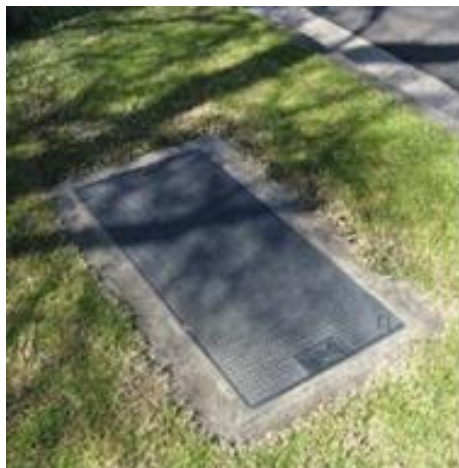
Figure 9 Underground housing for telecommunications facilities
