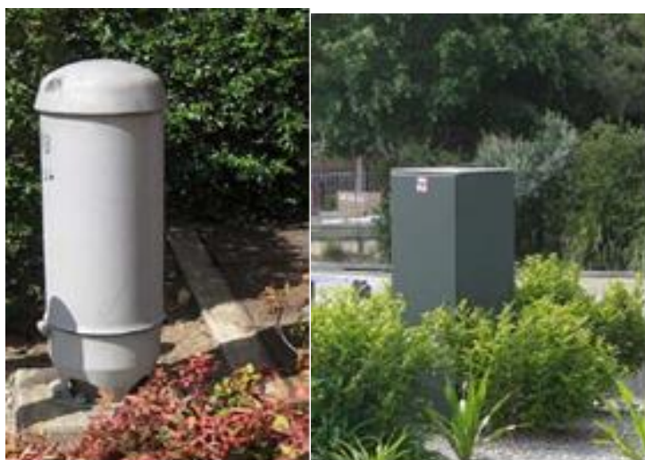
Figure 10 Left: Pillar Right: Cabinet
