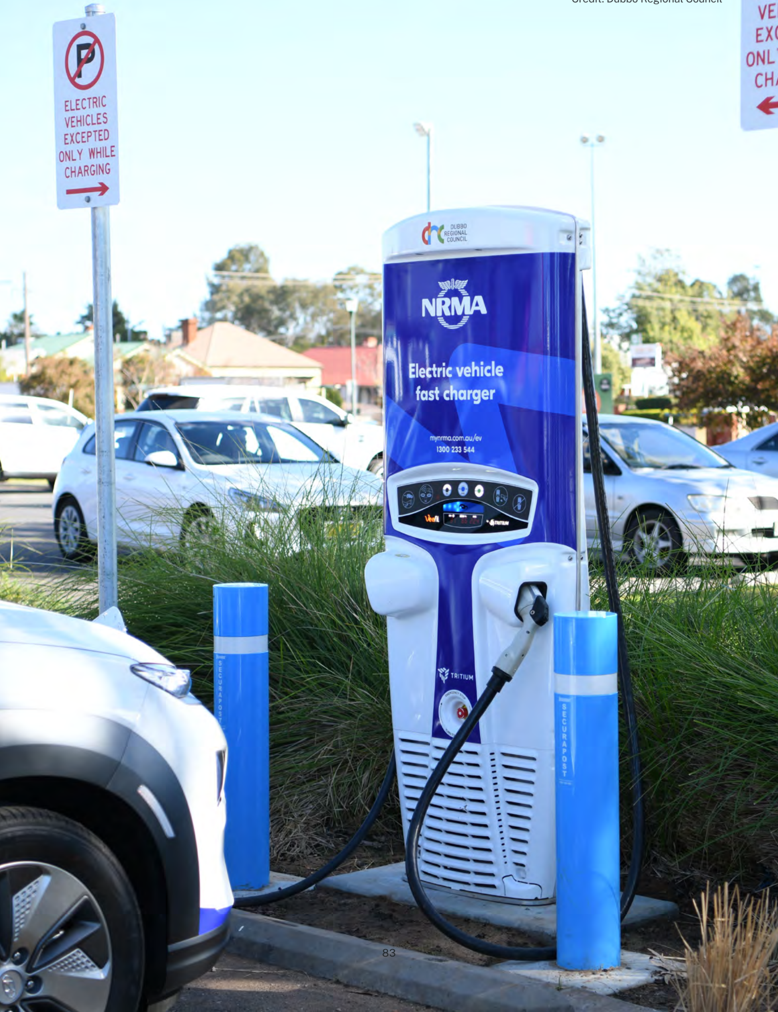
An electric vehicle charging station in Dubbo. Credit: Dubbo Regional Council
