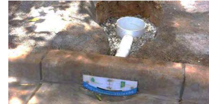
Example of Treenet infiltration trench. Source: Water By Design, Waterwise Street Tree Booklet
